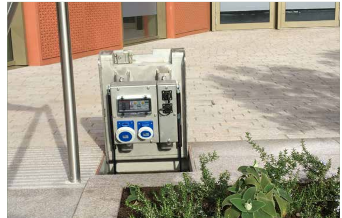
Use this box for Food Carts connecting cooking equipment. Can have 32 Amp 3 Phase Power for heavy use.
